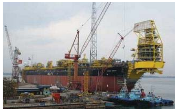
Figure-1. FPSO Kikeh under construction. Turret structure is shown on the bow of the vessel.
