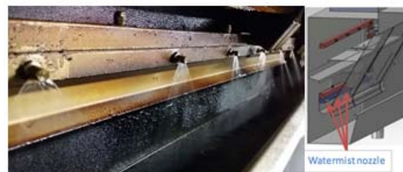
Figure-2. Water mist spray (mist curtain) operated.
