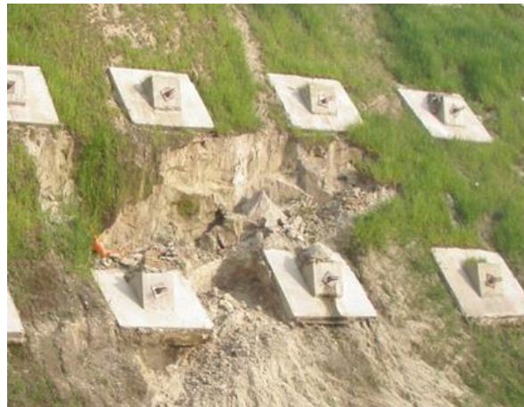
b) Erosion problems in areas not covered by individual concrete blocks.
