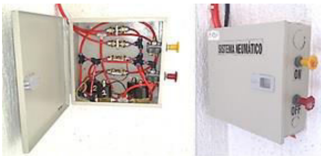
Figure-12. Pneumatic system control board.
