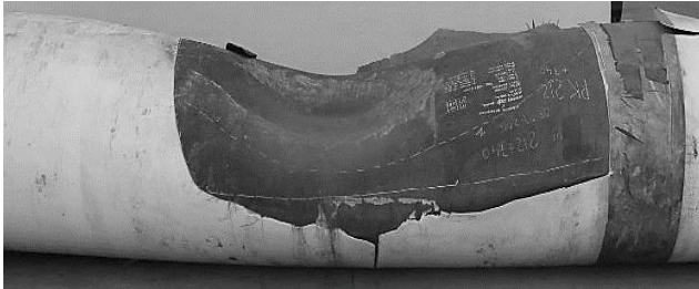
Figure-1. Pipe with buckling damage.
