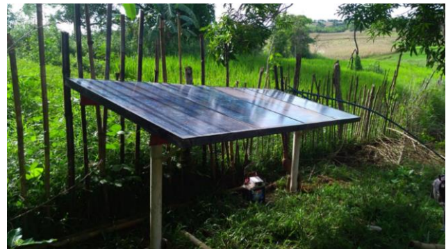
Figure-6. The power source of the electrical system.
