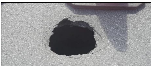
Figure-1. Cavity appearing underneath the road surface.
