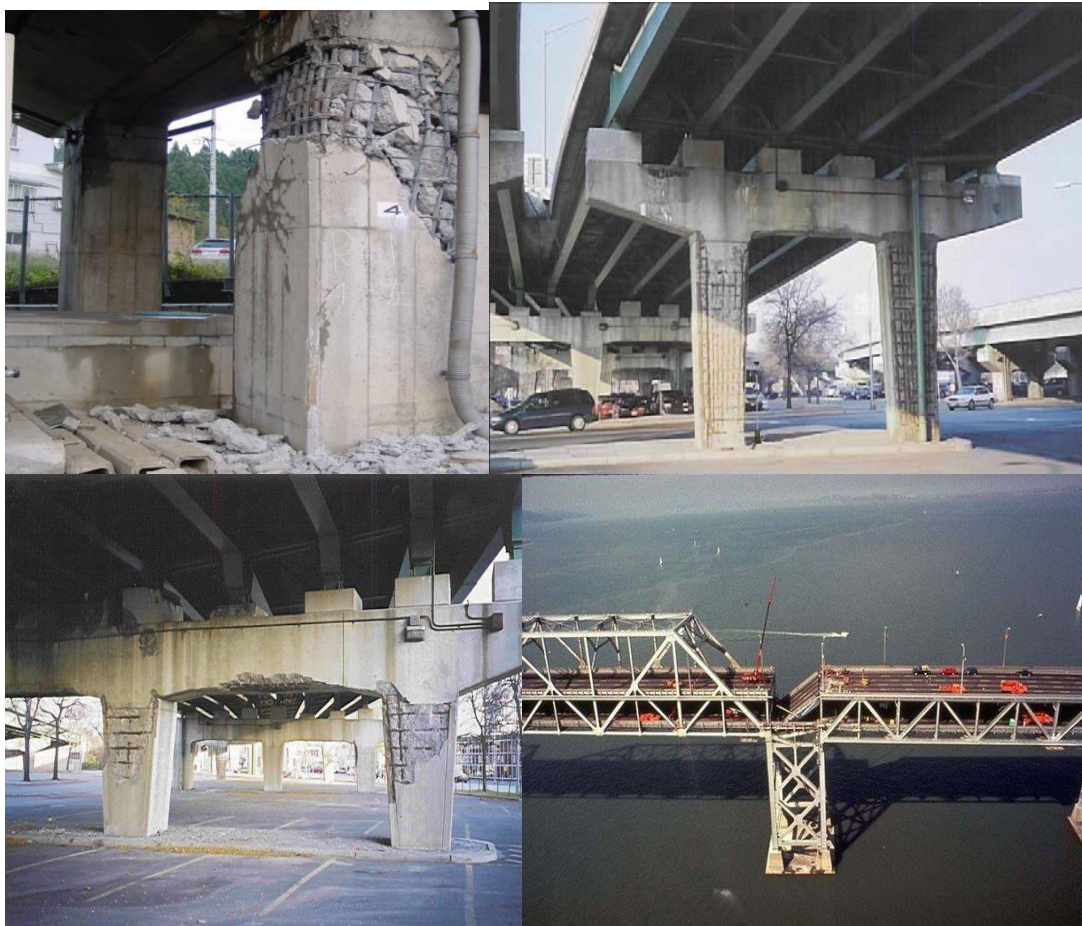
Figure-12. Damages of bridge structure [93].
