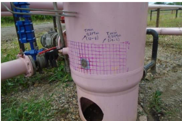
Figure-3. Verify minimum thickness in the lower zone of the separator's shell.
