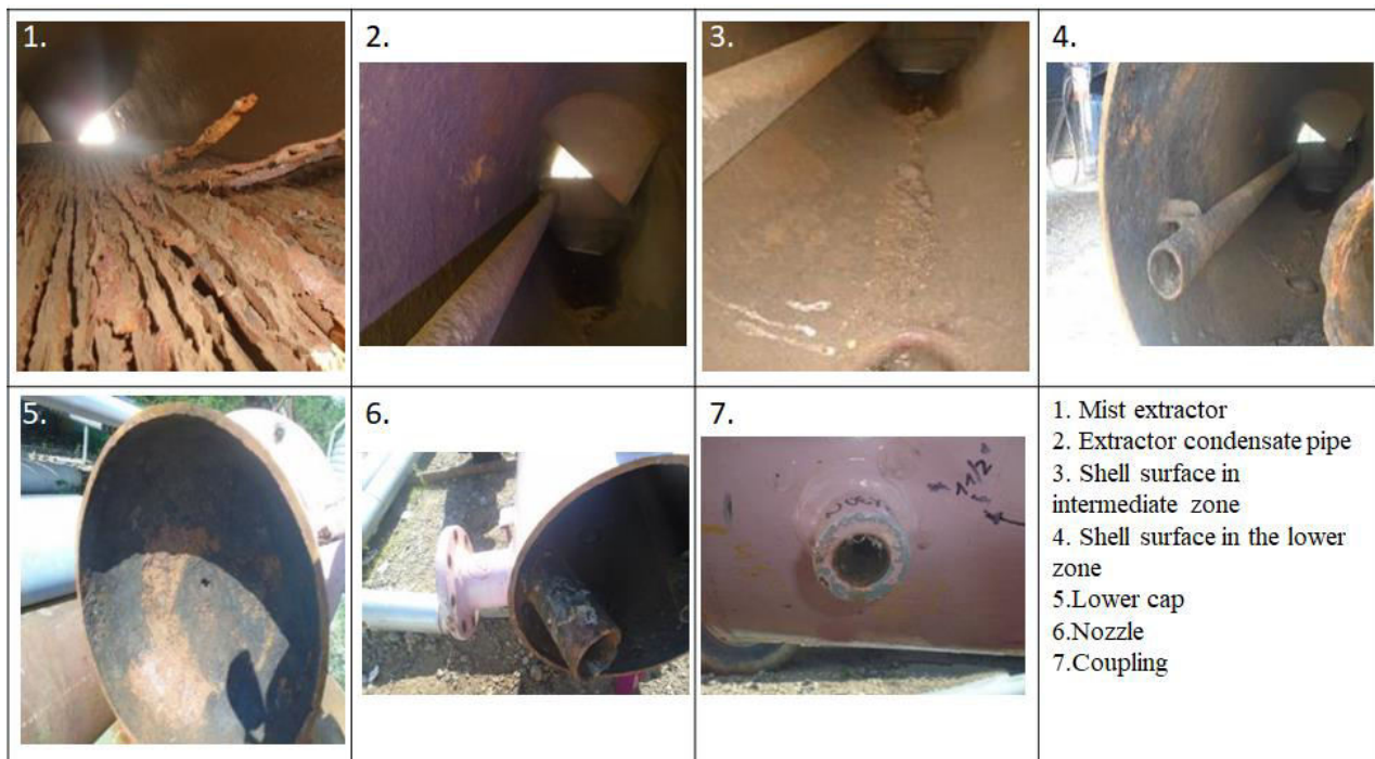
Figure-12. Photos of damage mechanisms in the internal part of the separator.
