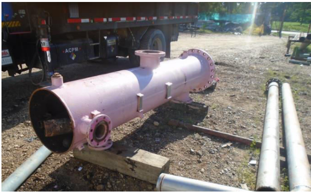
Figure-11. Disassembled TEA vertical two-phase separator for internal inspection.
