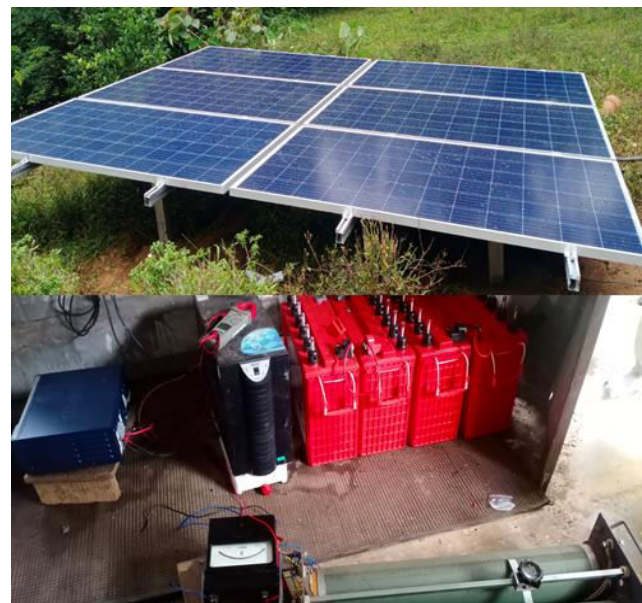
Figure-19. Experimental setup for 2KW solar PV system.
